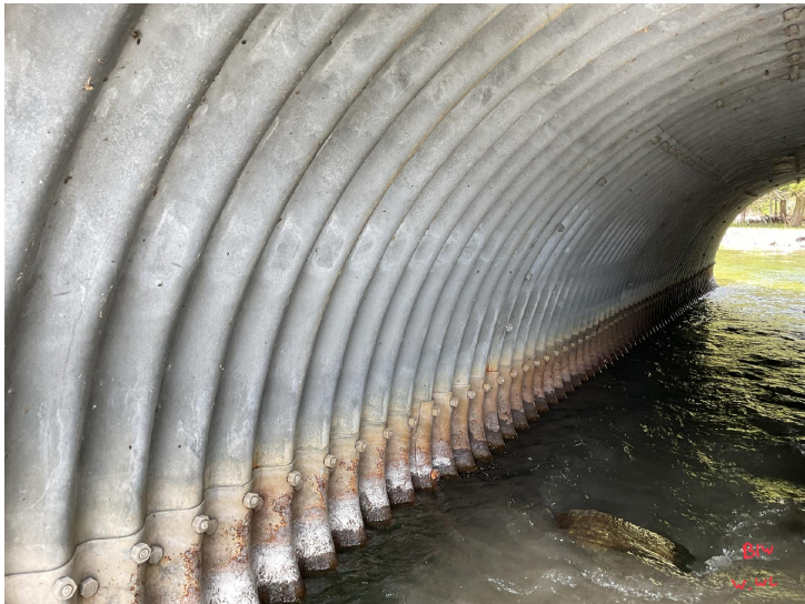
Document Name: IMG_0181.JPG Category: Culvert Span Number: Comments: Barrel 1W, west wall
