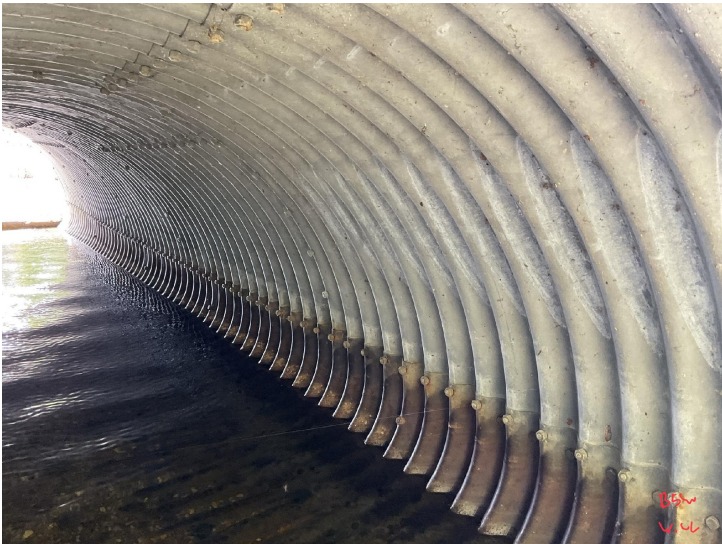
Document Name: IMG_0193.JPG Category: Culvert Span Number: Comments: Barrel 5W, west wall
