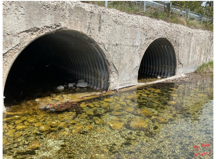
Document Name: IMG_0200.JPG Category: Channel Span Number: Comments: Timber debris blocking inlet of barrels 4W & 5W
