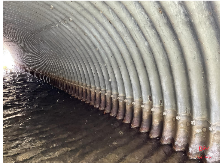
Document Name: IMG_0184.JPG Category: Culvert Span Number: Comments: Barrel 2W, west wall
