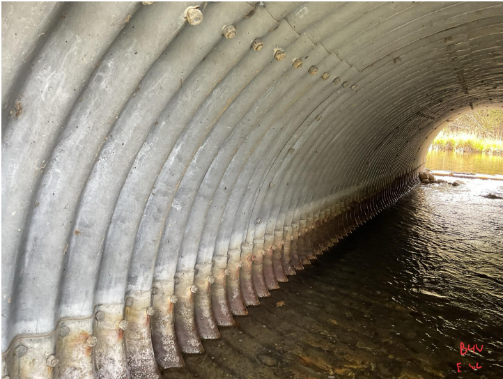
Document Name: IMG_0191.JPG Category: Culvert Span Number: Comments: Barrel 4W, east wall
