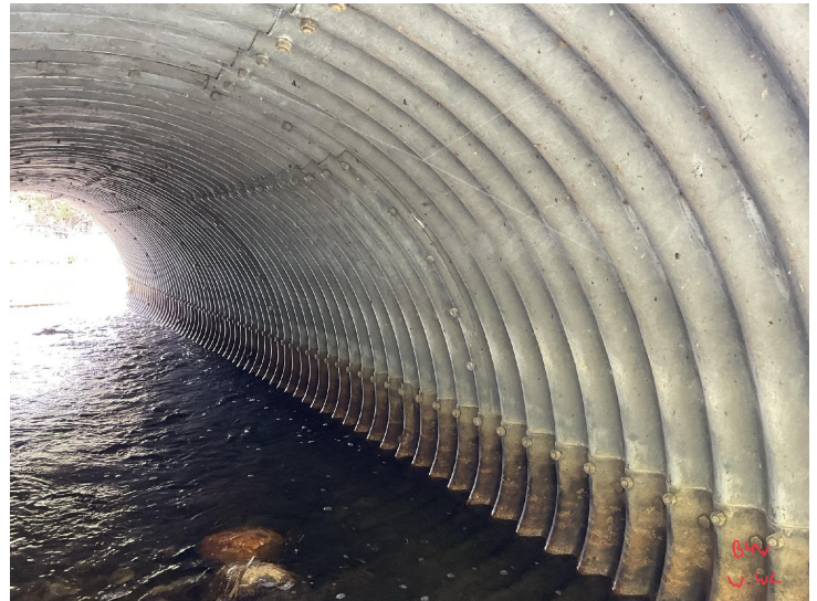
Document Name: IMG_0190.JPG Category: Culvert Span Number: Comments: barrel 4W, west wall
