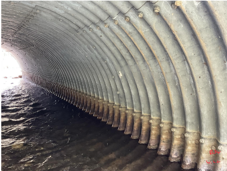
Document Name: IMG_0187.JPG Category: Culvert Span Number: Comments: Barrel 3W, west wall
