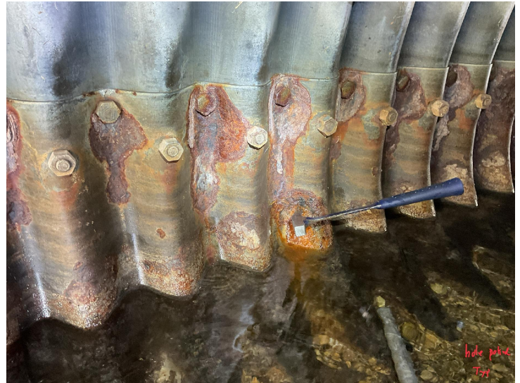
Document Name: IMG_0196.JPG Category: Culvert Span Number: Comments: Hole poked, typical
