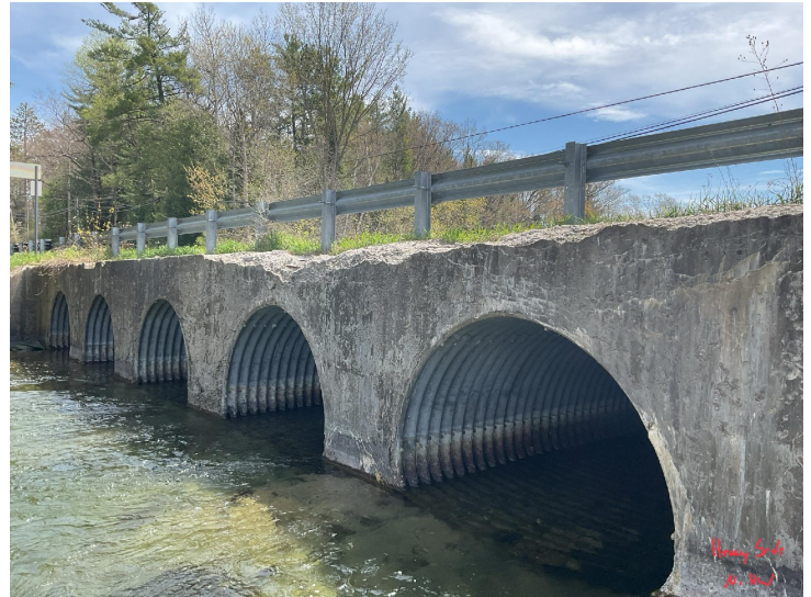
Document Name: IMG_0199.JPG Category: Culvert Span Number: Comments: Heavy scale in north headwall
