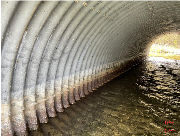
Document Name: IMG_0185.JPG Category: Culvert Span Number: Comments: barrel 2W, east wall
