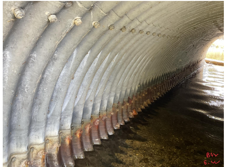
Document Name: IMG_0194.JPG Category: Culvert Span Number: Comments: Barrel 5W, east wall
