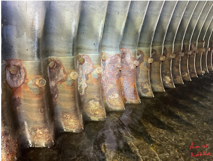
Document Name: IMG_0197.JPG Category: Culvert Span Number: Comments: Area of heavy rust and scale
