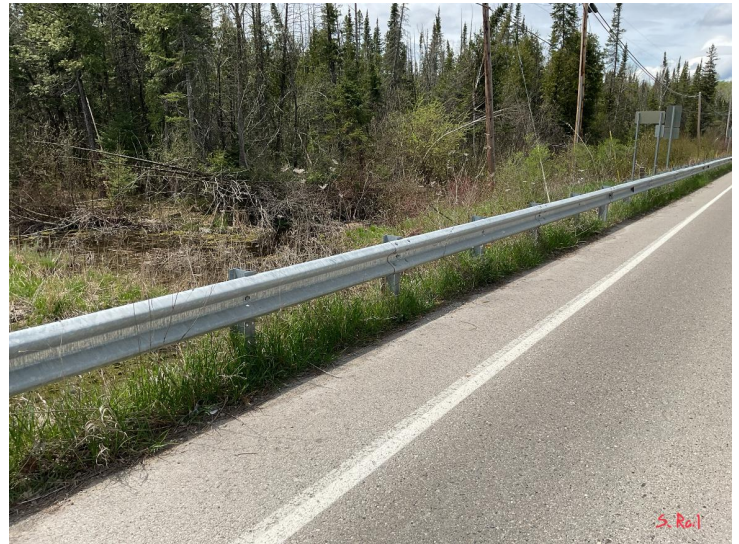
Document Name: IMG_0176.JPG Category: Railing Span Number: Comments: South rail
