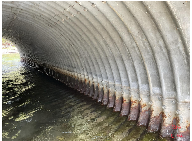
Document Name: IMG_0182.JPG Category: Culvert Span Number: Comments: Barrel 1W, east wall
