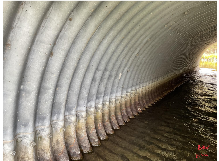
Document Name: IMG_0188.JPG Category: Culvert Span Number: Comments: Barrel 3W, east wall
