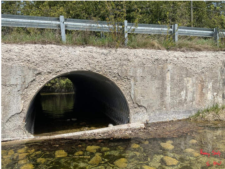
Document Name: IMG_0201.JPG Category: Culvert Span Number: Comments: Heavy scale in south headwall
