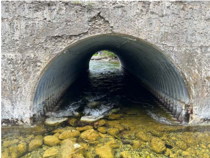
Document Name: IMG_5669 conv.jpeg Category: Culvert Span Number: Comments: Barrel 3W from S
