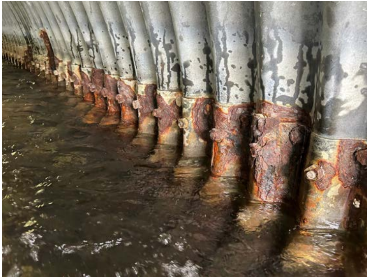
Document Name: IMG_5680 conv.jpeg Category: Culvert Span Number: Comments: Barrel 5W, E wall, scale at WL
