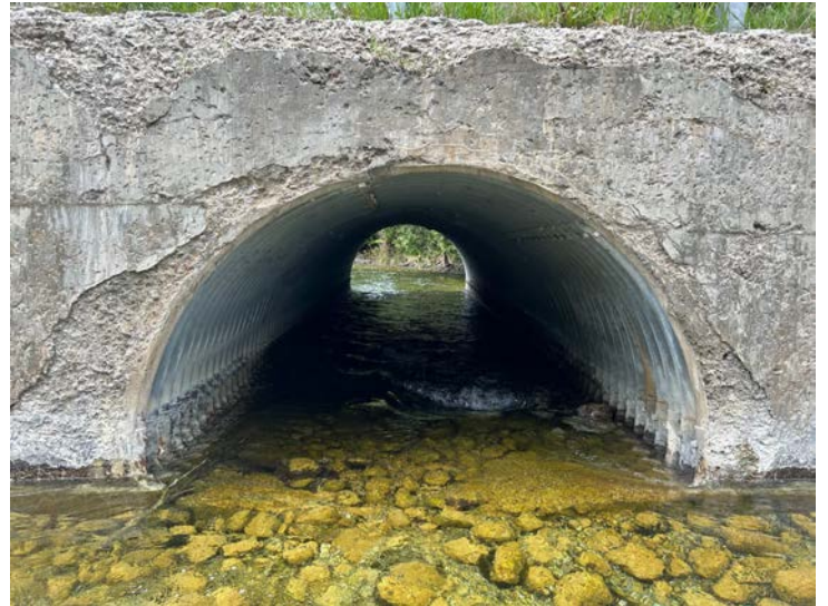
Document Name: IMG_5670 conv.jpeg Category: Channel Span Number: Comments: Barrel 4W from S
