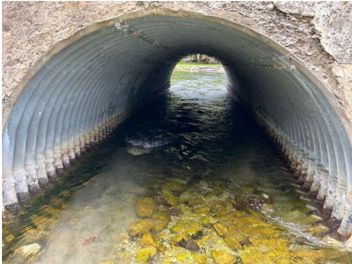
Document Name: IMG_5667 conv.jpeg Category: Culvert Span Number: Comments: Barrel 1W from S
