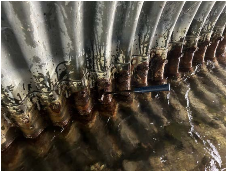
Document Name: IMG_5674 conv.jpeg Category: Culvert Span Number: Comments: Barrel 4W, E wall, hammer in hole - typ.
