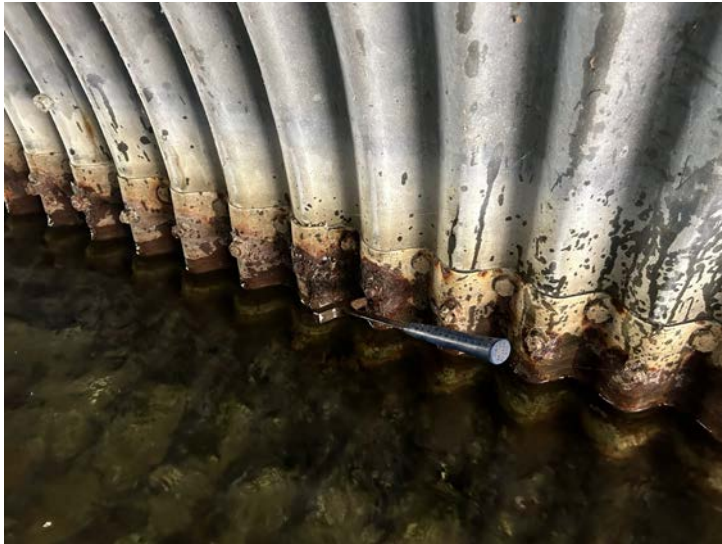
Document Name: IMG_5672 conv.jpeg Category: Culvert Span Number: Comments: Barrel 2W, E wall, hammer in hole - typ.
