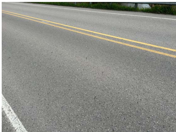
Document Name: IMG_5688 conv.jpeg Category: Deck Span Number: Comments: Deck surface - typ.
