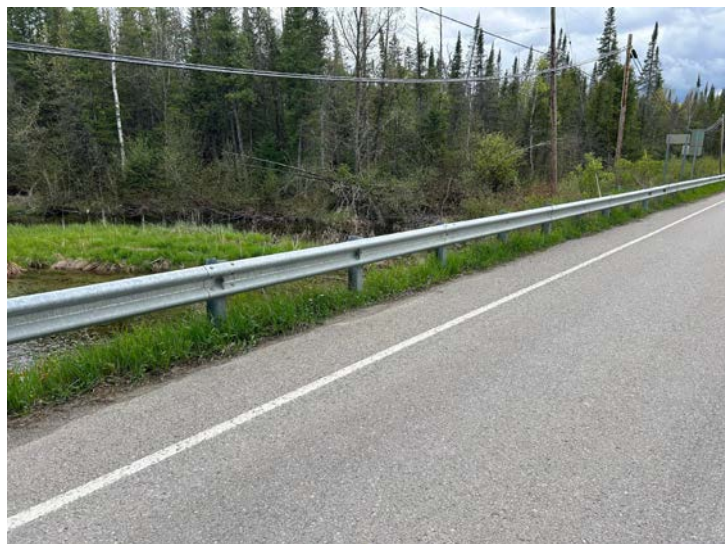
Document Name: IMG_5684 conv.jpeg Category: Railing Span Number: Comments: S rail
