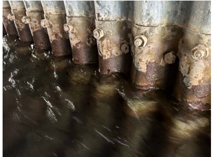
Document Name: IMG_5673 conv.jpeg Category: Culvert Span Number: Comments: Barrel 2W, E wall, existing holes - typ.
