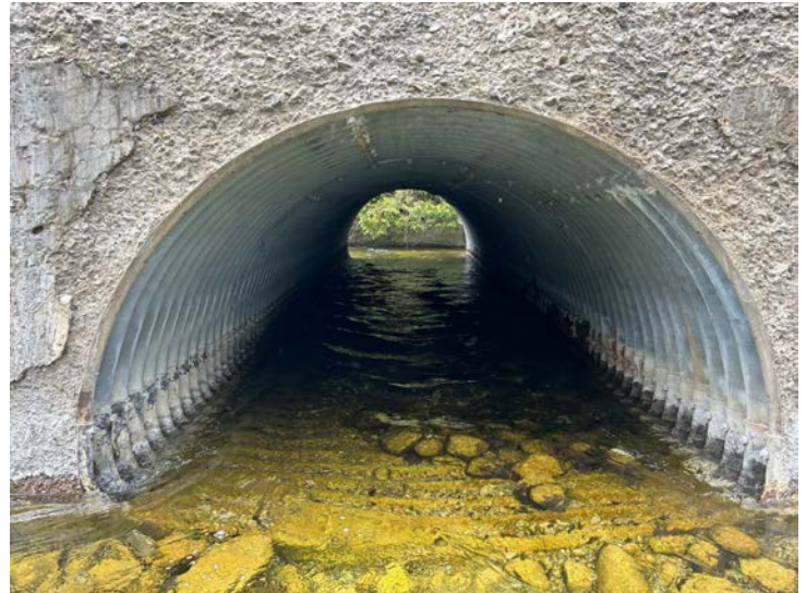
Document Name: IMG_5671 conv.jpeg Category: Culvert Span Number: Comments: Barrel 5W from S
