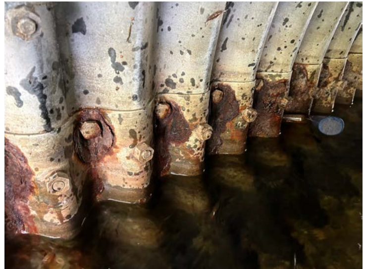
Document Name: IMG_5676 conv.jpeg Category: Culvert Span Number: Comments: Barrel 5W, W wall, scale at WL
