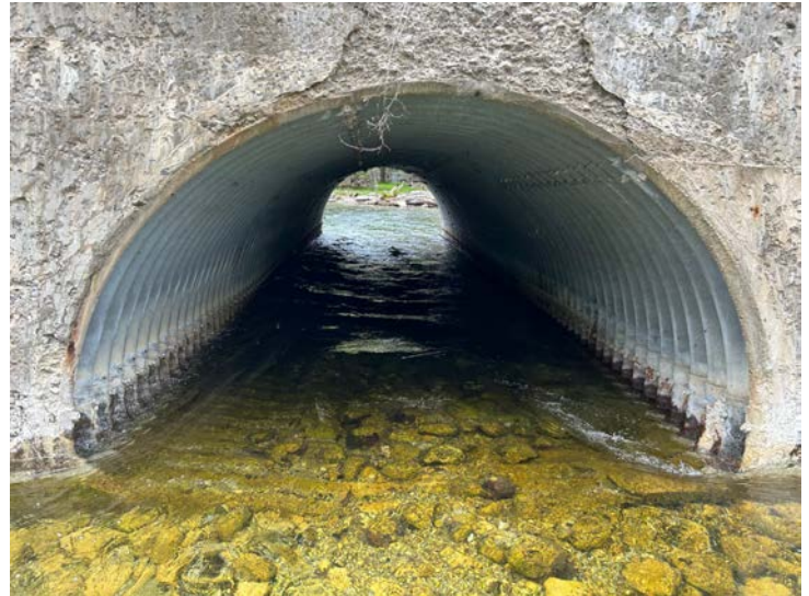
Document Name: IMG_5668 conv.jpeg Category: Culvert Span Number: Comments: Barrel 2W from S
